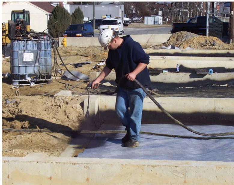
A synthetic barrier with the application of a spray-on impermeable sealer within a townhouse's foundation.
