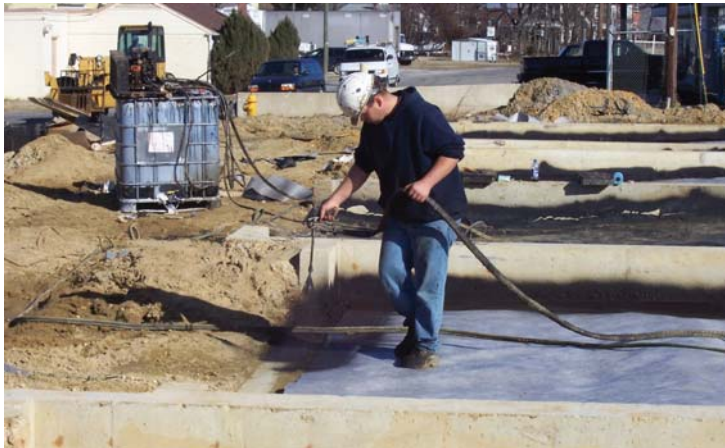
View of a synthetic vapor barrier with the application of a spray-on impermeable sealer within a townhome's foundation.
